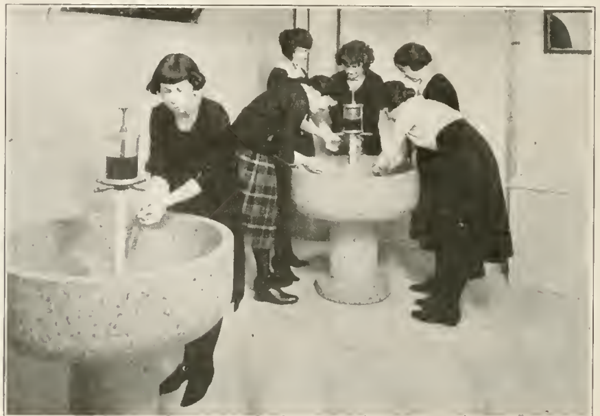
Hygienic, attractive in design, and economical in space and the number accommodated, is this washfountain built of highly polished ground marble and concrete. The water is controlled either by a foot or hand lever with soap containers as part of the construction. The installation is used in railway stations, public buildings, and industries where large numbers must wash in a short time.
